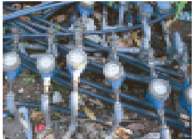
SSWPs often use meters to manage
