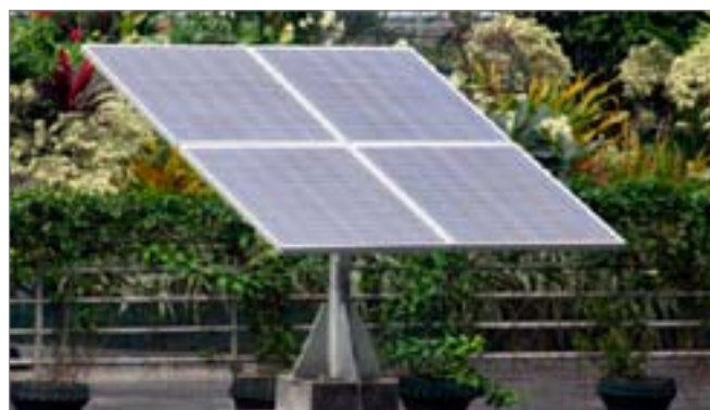
Solar energy for a fountain, by a roof-top garden.
