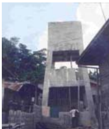
Water tower of small pipe system in Cebu
