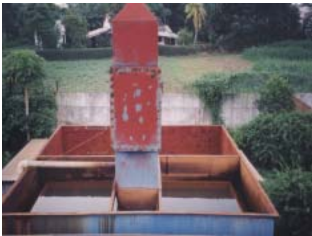
Water treatment unit implemented in Ho Chi Minh City (Phuc Doan Company)
