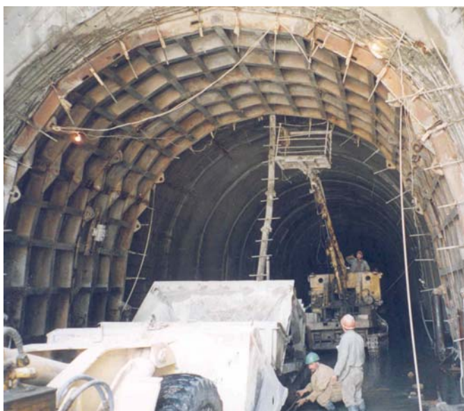
WORKING FOR PROGRESS Construction of tunnels for better transport system through public-private sector partnership
