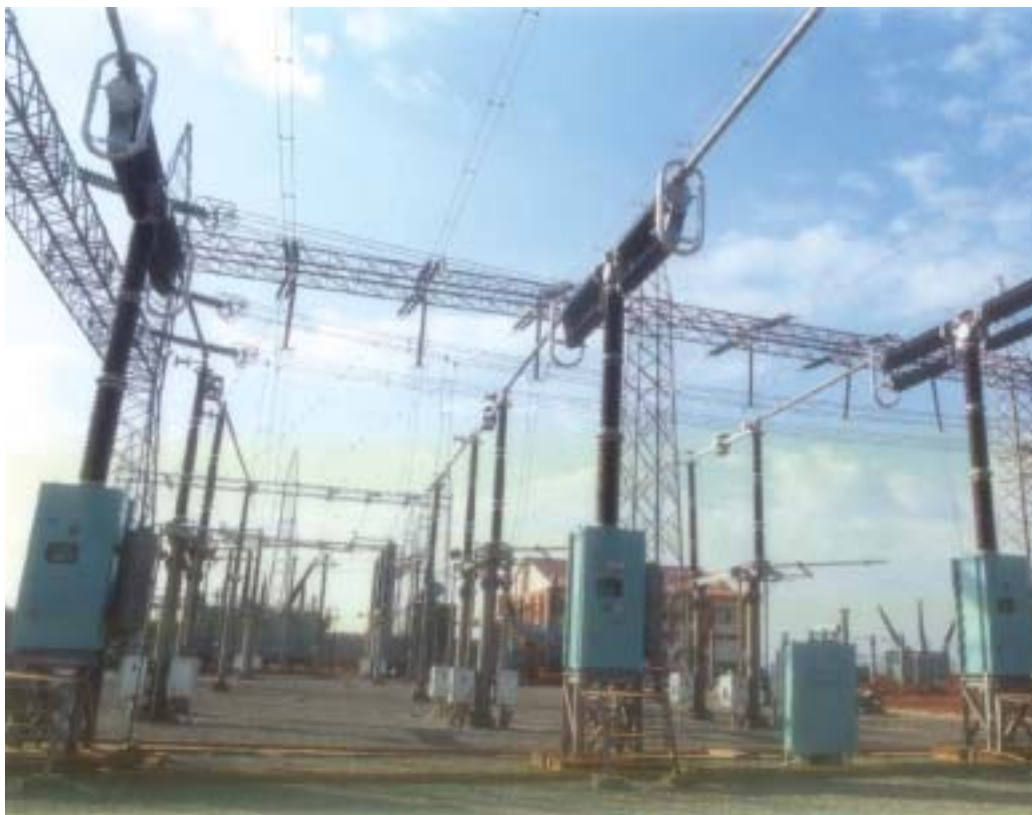
View of ADB funded Mapusa 400/220 kV substation switchyard
