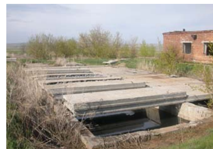
PHYSICAL INFRASTRUCTURE IN RURAL AREAS Water storage reservoirs in Pavlodar oblast to be upgraded and rehabilitated under the project
