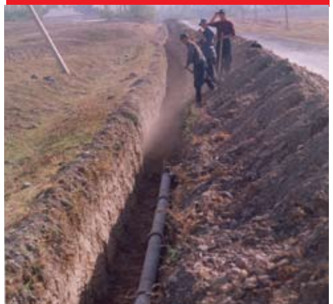
ADB's Community-Based Infrastructure Services Sector Project provides piped drinking water to people in rural areas
