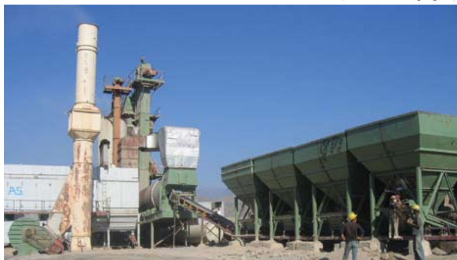
A mobile asphalt plant in Tash-Kumyr located along the reconstructed parts of the Bishkek-Osh road
