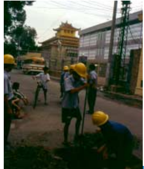
BASIC INFRASTRUCTURE An ADF project helps improve the urban environment in Ho Chi Minh City, Viet Nam
