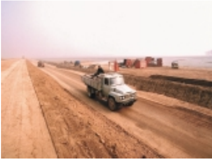
Construction of the Hebei Roads Development Project 河北公路项目的建设现场
