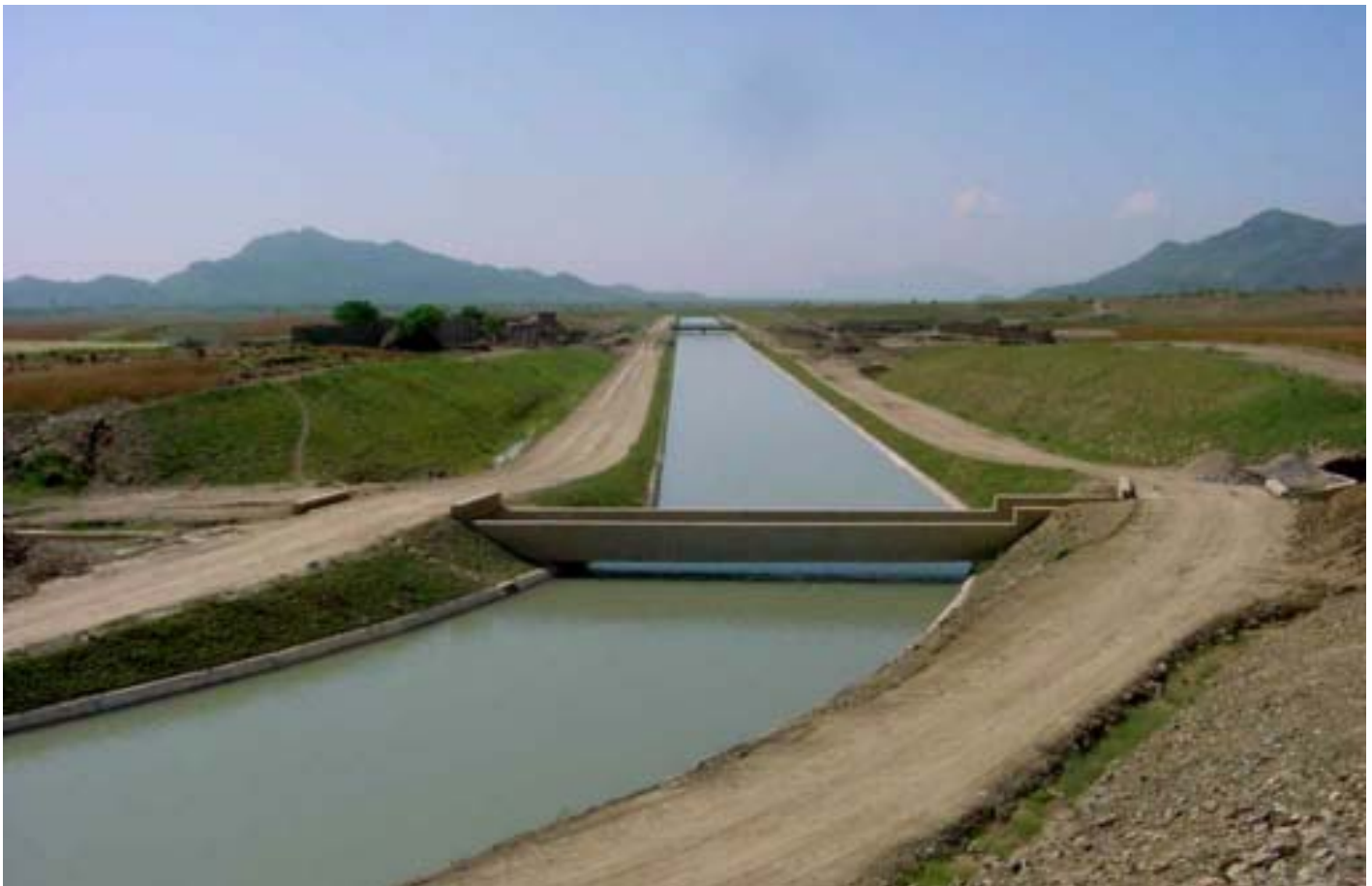
IMPROVING IRRIGATION A parabolic canal constructed under Pehur high-level canal project in North West Frontier Province
