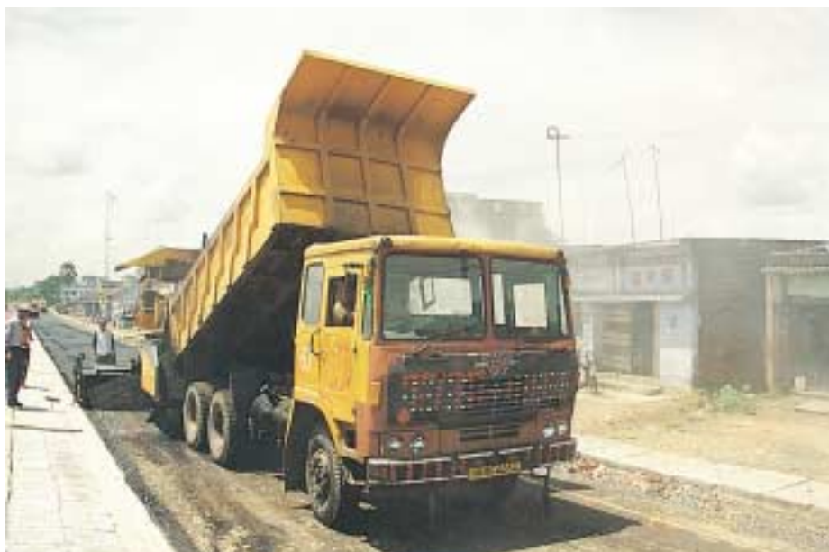
The National Highway Authority of India is constructing four-lane highways and strengthening existing two-lane roads
