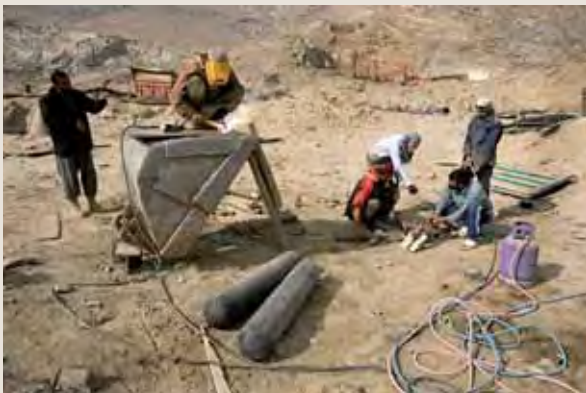
Construction companies are among local businesses benefiting from ADB-backed Afghanistan International Bank loans
