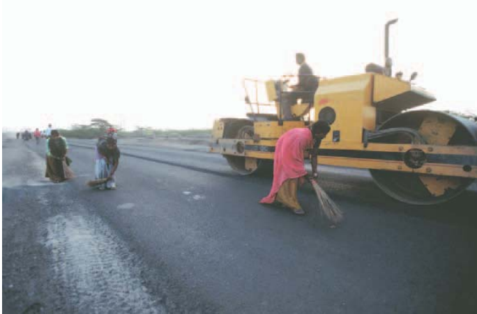
One way of increasing the poverty reduction impact of road construction is to employ the poor as laborers, as in this project near Mundra, Gujarat State, India.
