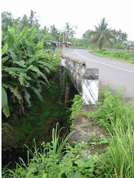
Alue Ketapang - Bridge to be replaced
