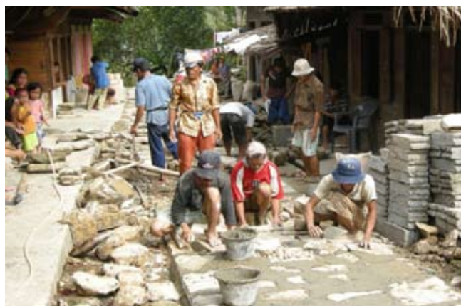
A community contract in progress: many hands lay the path for improved village infrastructure.
