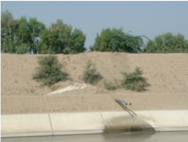
Breached section of embankment near Vehowa culvert-1
