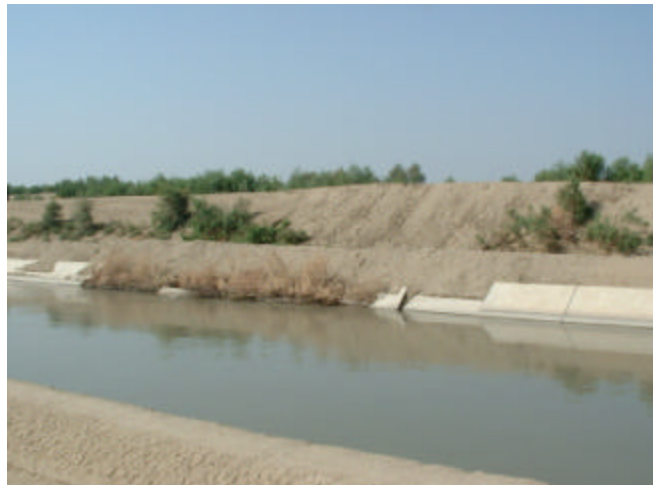
Breached section of embankment near Vehowa culvert-4, (canal lining was also damaged)
