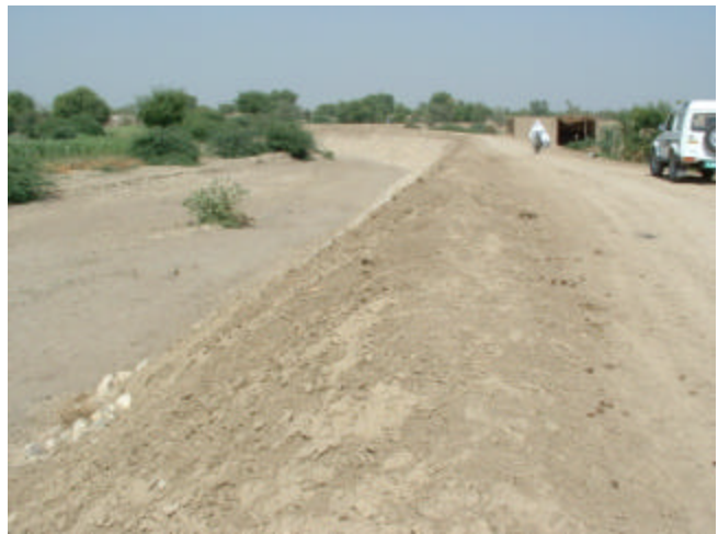
Eroded section of the protection bund of Sokkar
