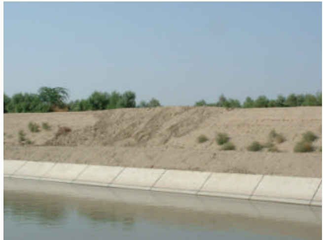
Breached section of embankment near Vehowa culvert-2
