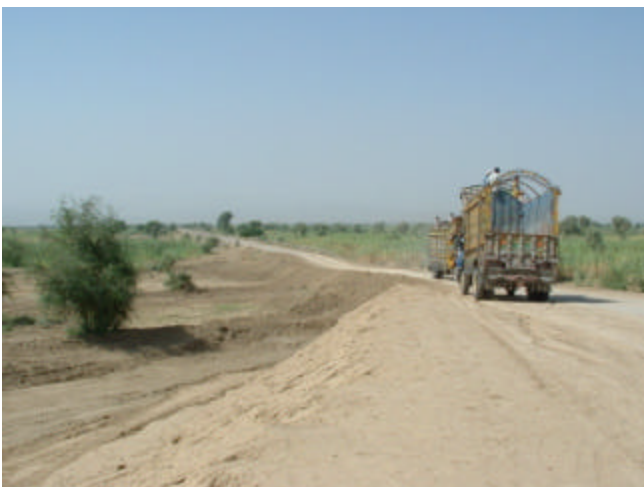
Breached road due to floods (at RD804)
