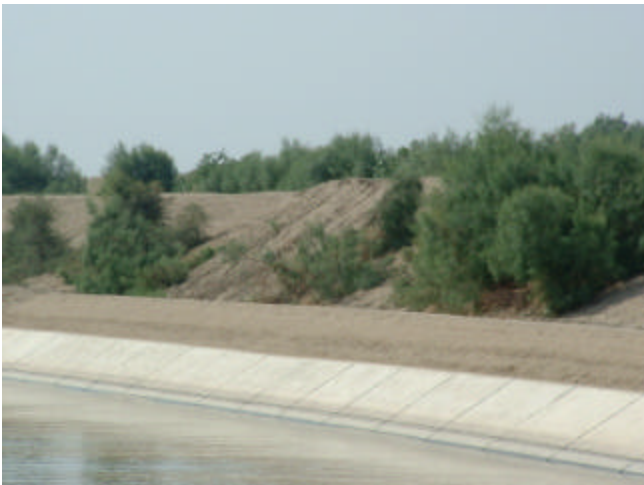
Breached section of embankment near Vehowa culvert-3
