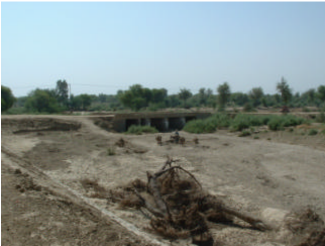
Bridge in Sokkar that caused erosion of protection bund
