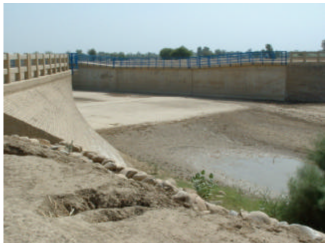
Bughlani superpassage: leveled sill due to siltation
