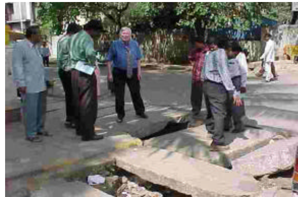
Bob Hood with Bangalore coordinators inspect one of the on-going trenching works.
