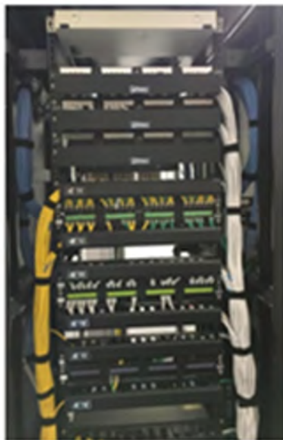
Sample Cabling Management
