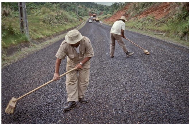
Men laying asphalt on a road in Fiji, which is part of the Road Maintenance Sector Project. Roads in ADF countries are rated as in poor condition overall, but varying by country.
