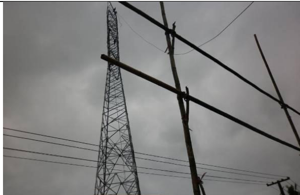
Photos 5: Scaffolds were also used to prevent the affect on the local electric system
