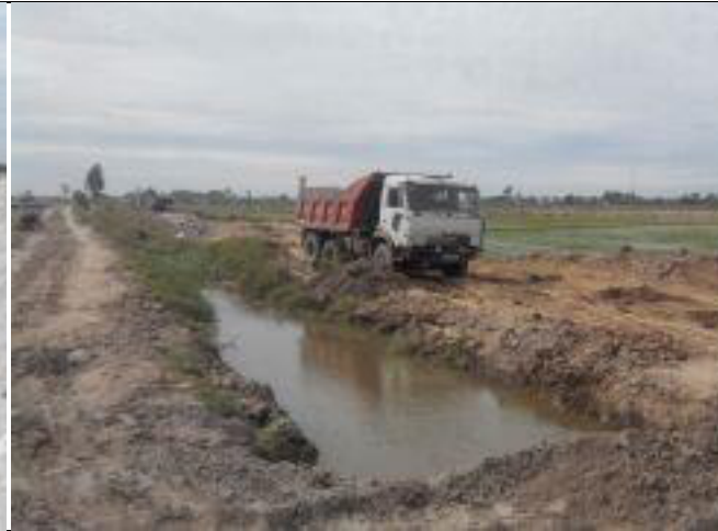
Photos 2: Material on the truck has been covered to prevent the air pollution
