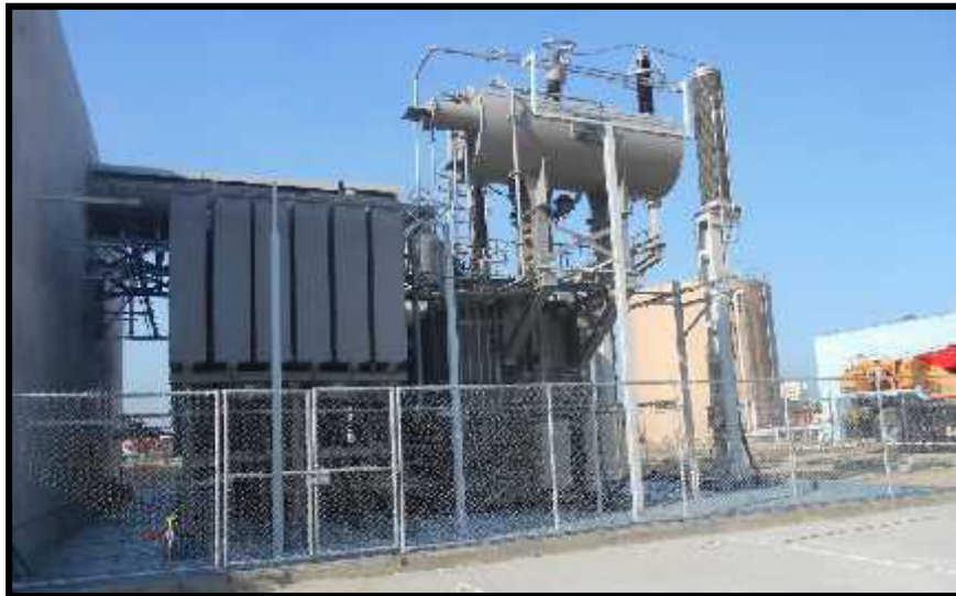
STEP UP TRANSFORMER
