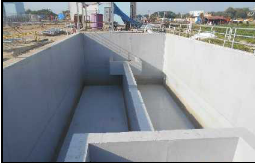
WASTE WATER TREATMENT PLANT
