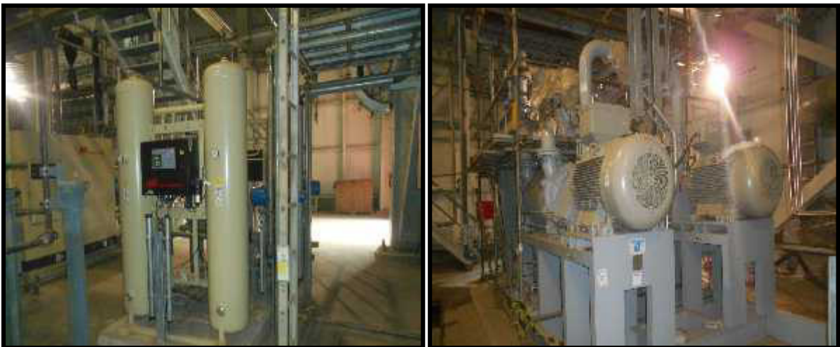
COMPRESSED AIR SYSTEM
