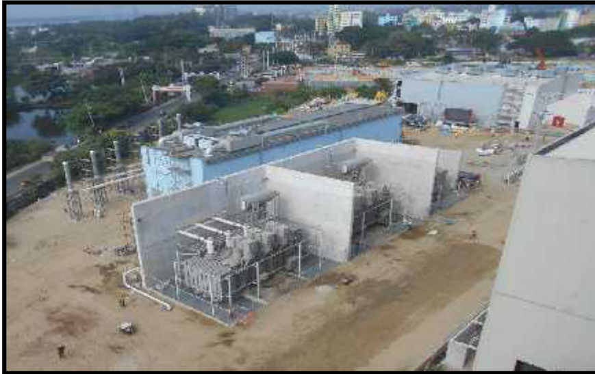
GAS TURBINE AREA
