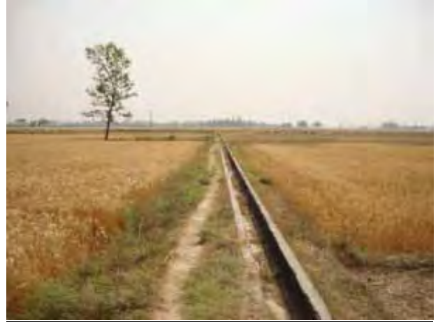
Km 0+700 - Existing brick lined irrigation canal where 90 dia pipe culvert has been proposed.
