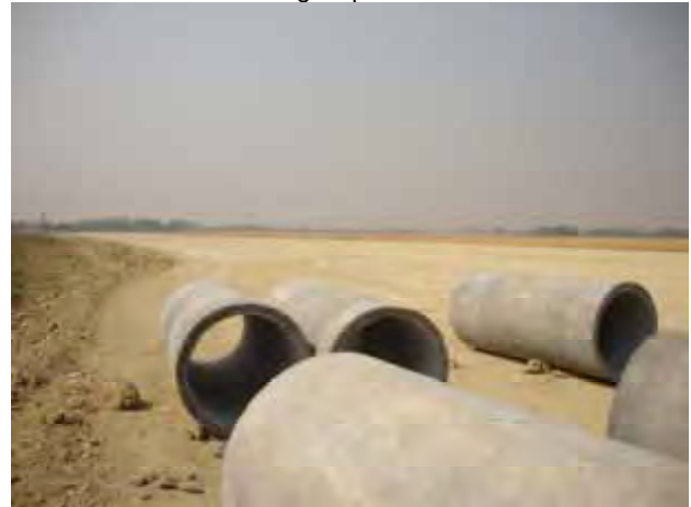
Road side parking area under construction for vehicles awaiting Custom clearance besides starting point of BBY Road.
