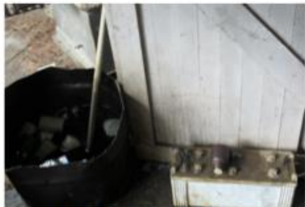
Existing practices for used oil and battery management in Mauke powerhouse need immediate attention
