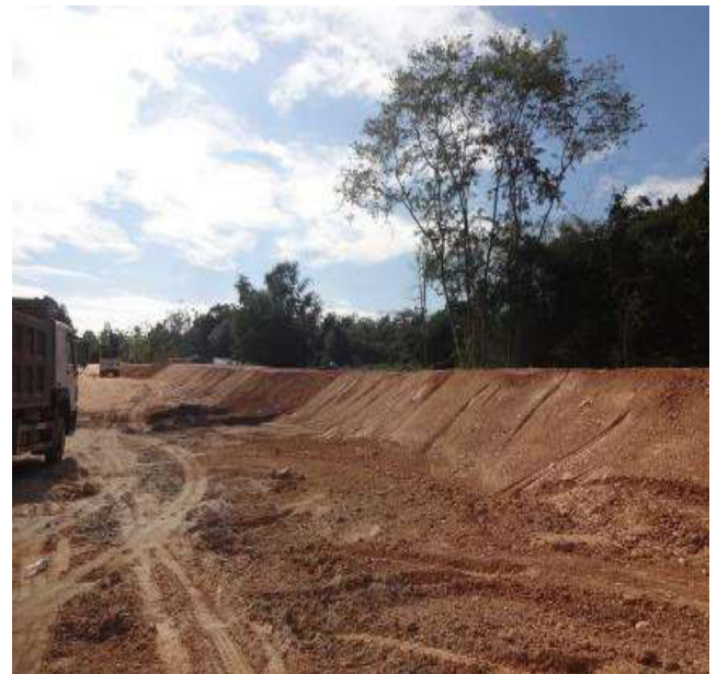
Plate 8: The barren slope of the main canal embankment needing grasses or any vegetative cover as soil conservation measure
