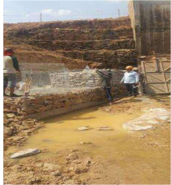
Plate 2: Concrete rapping of stone wall for the box culvert approach along the road-dike
