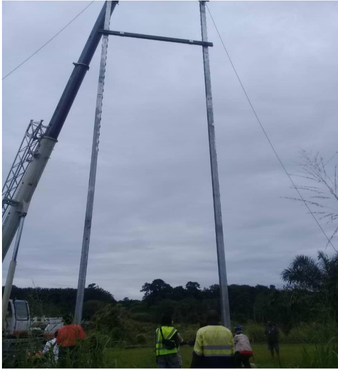
Erection of 2x H Frames for conductor stringing across the 500m Kumusi Bridge- Oro Province
