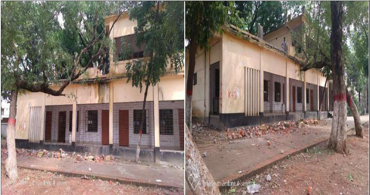
Photos of on-going demotion works of the existing school building where the CCS rooms will be constructed (As of 30 April 2018)
