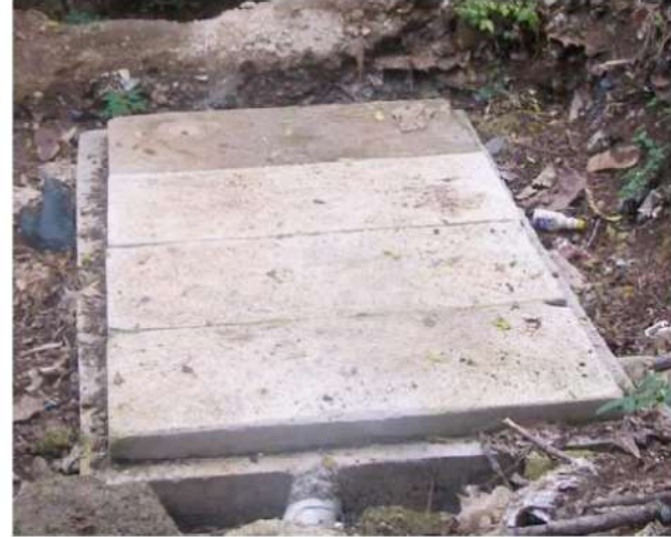
Community drop toilets are being replaced with new facilities and septic systems (under construction above)
