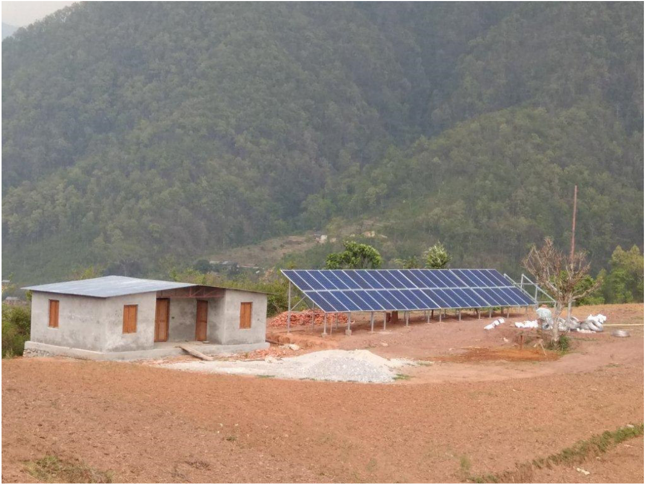
Power house and ground mounted solar panel at Chisapani, Sindhuli
