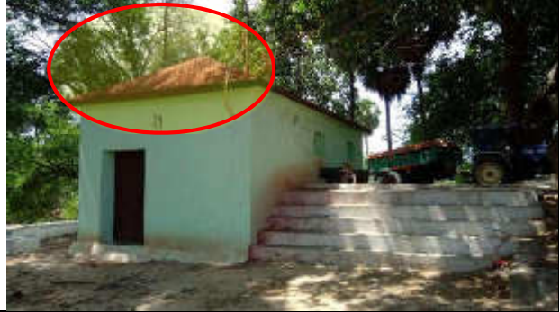
Construction is not properly completed. The steel rods are not completely removed
