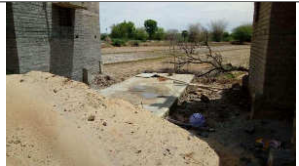
Septic Tank is provided
