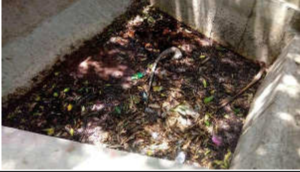
Periodic Cleaning is not done
