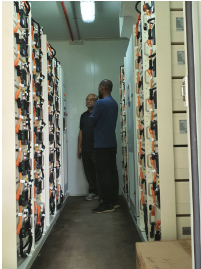
Figure 7. Inside a BESS unit
