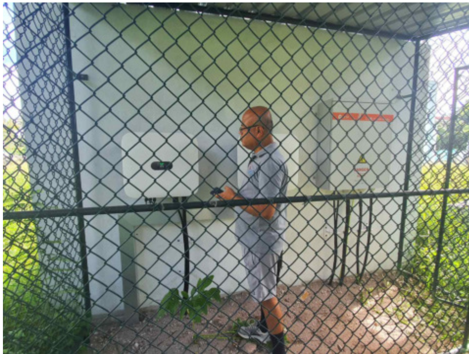
Figure 5. Inverter room in Nolhivaram
