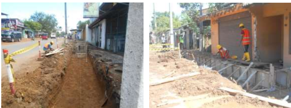
Figure:3.2 The improvement works are started in the Moratuwa-Piliyandala road and line drains are being constructed.
