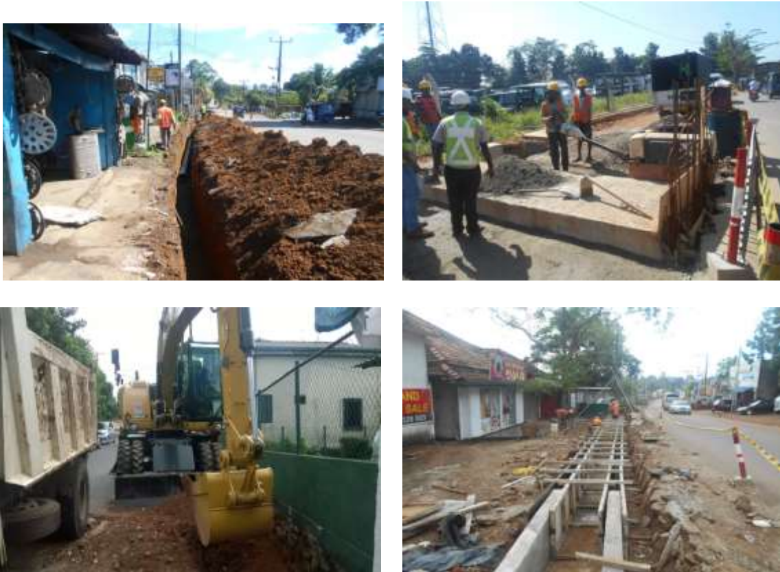
Figure 3.1 The ongoing works on Pipe laying, drain construction and Culvert work of Rathmalana-Mirihana road(B386)
