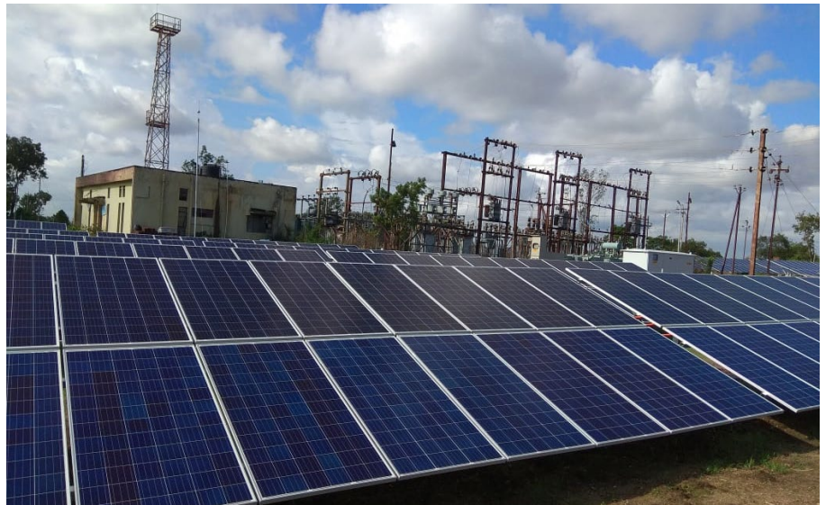
Distributed solar photovoltaic system set up by EESL
