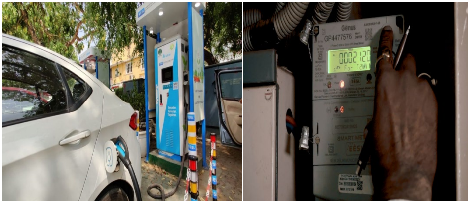
An electric vehicle charging station and (right) an installed smart meter
