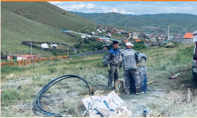
Workers conducting test drilling for the ground source heat pumps to be deployed in Ulaanbaatar, Mongolia (photo by ADB).
