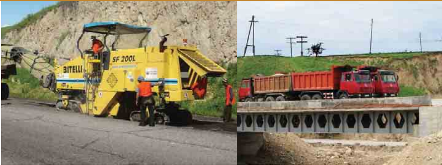
Milling (left) and load testing (right), Dushanbe–Kyrgyz Border Road Rehabilitation Project (Phase III)
